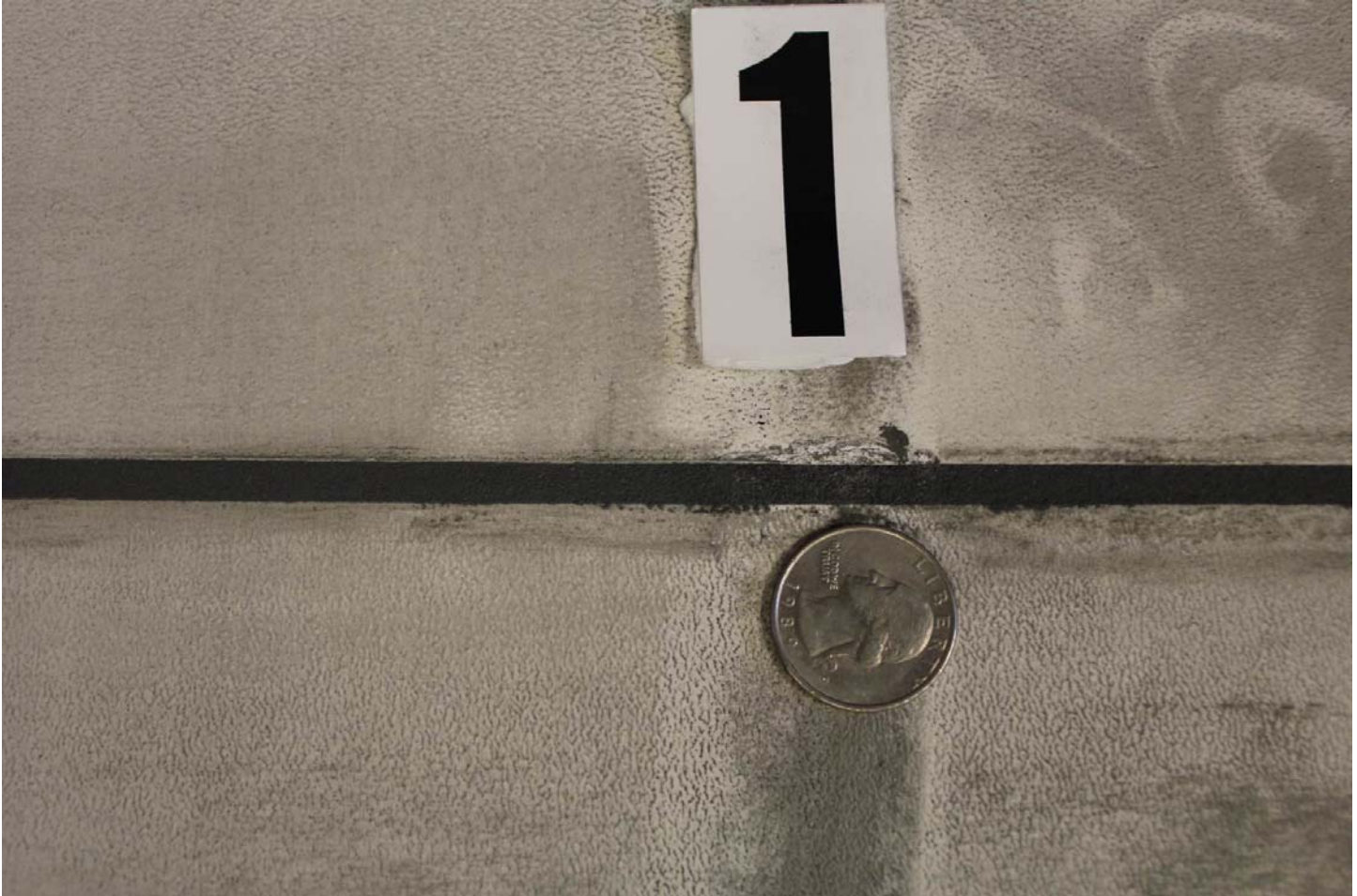
Image 2: Chipped tile at grout joint labeled “1” in figure 1. The damage took place during cycle fourteen.
