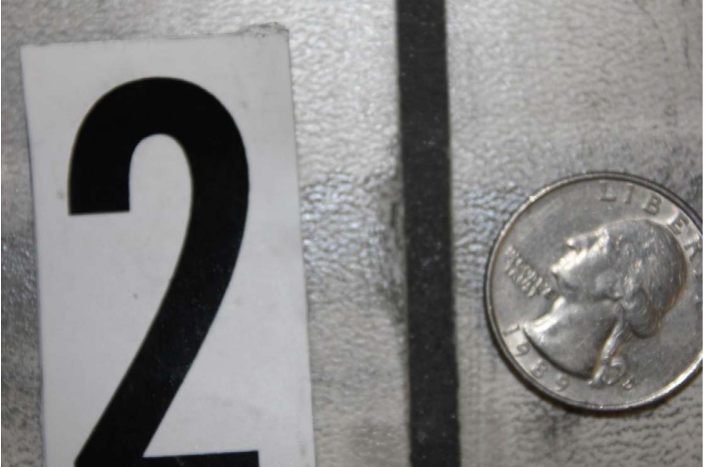
Image 2: Chipped tile at grout joint labeled “2” in figure 1. The damage took place during cycle fourteen.
